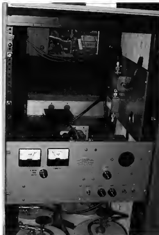
Figure 4—An inside view of the WIKKF repeater. The controller takes center stage, while the duplexer is visible at the bottom of the cabinet.
